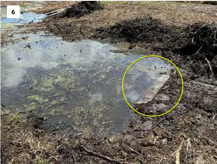
Mitered end 3 of 3 Was under water, but you can see the top edge.
